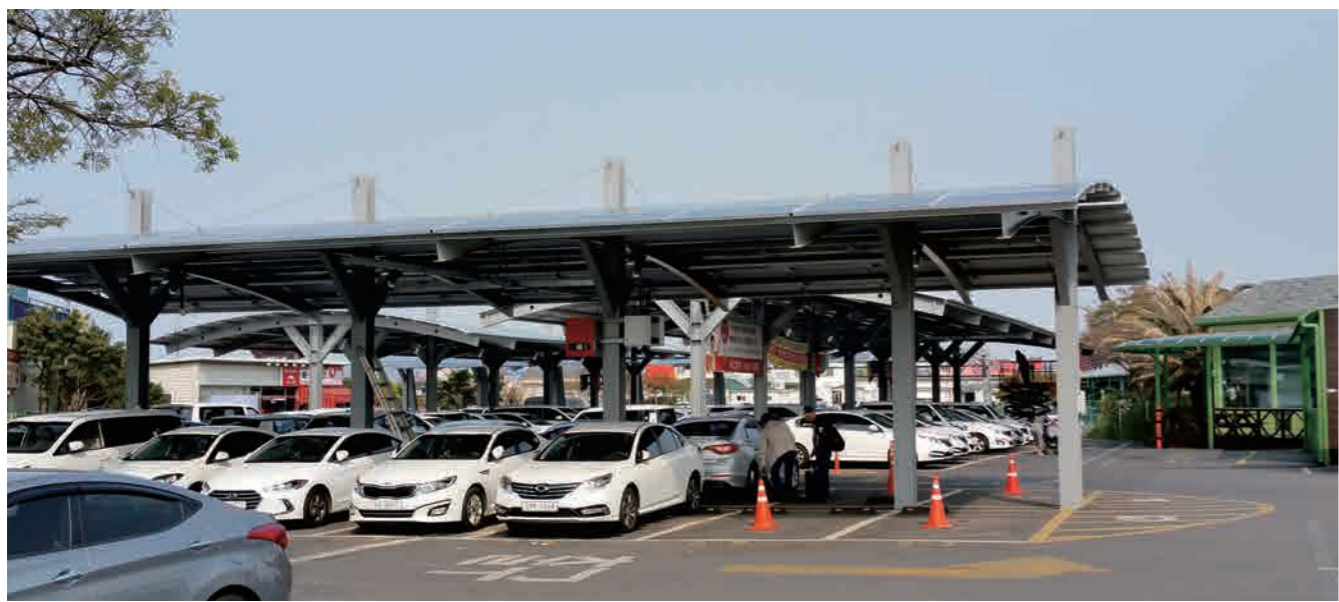
185kW, PV Carport, South Korea
