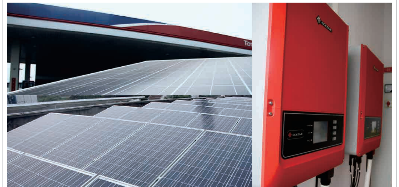
30kW, Petrol station
