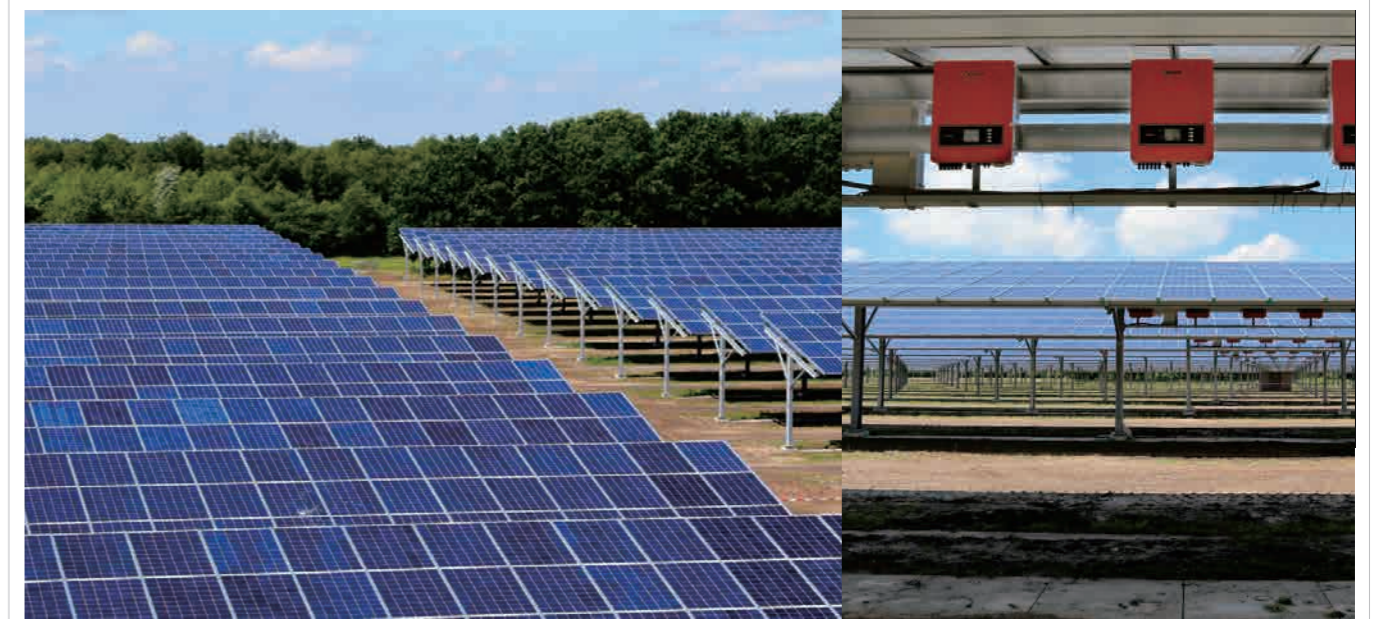
5MW, the Netherlands
