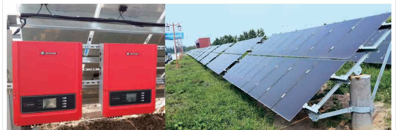
250kW, Shangdong, China
