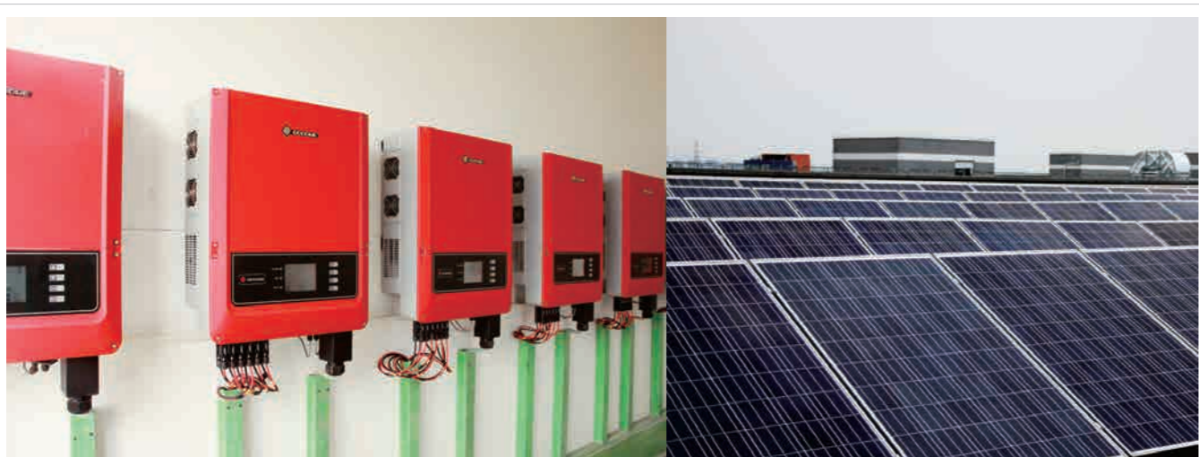
500kW, Shanghai, China
